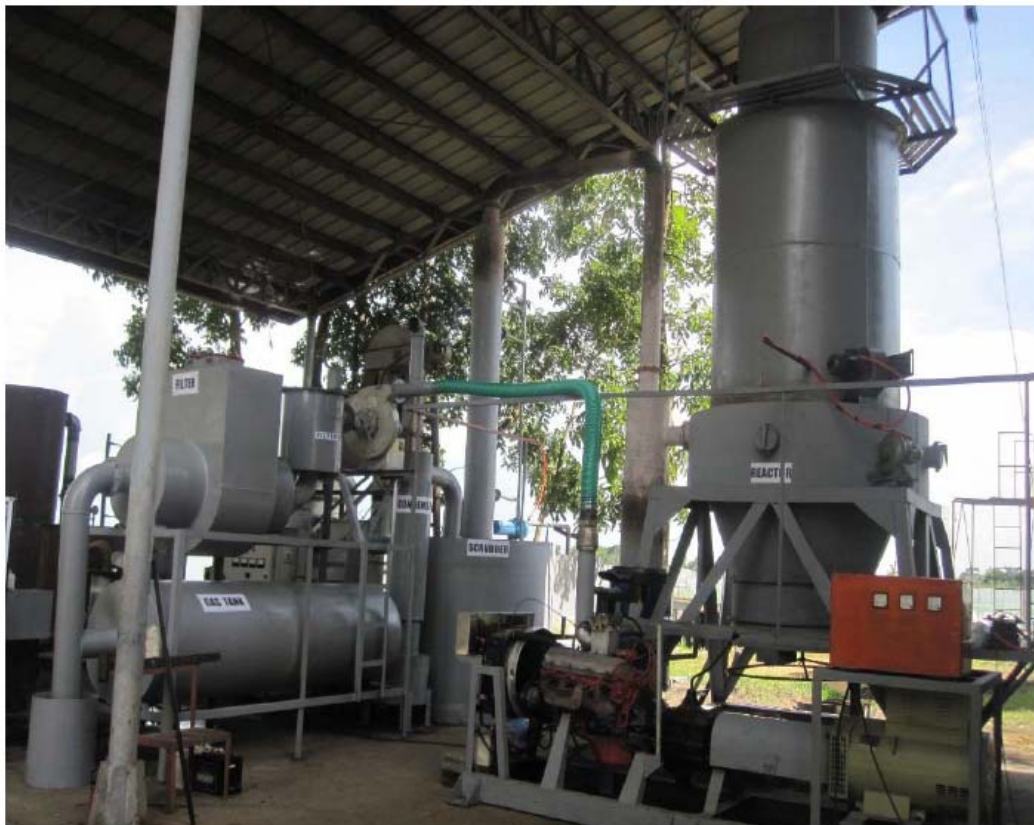
The 100-kWe Plant
