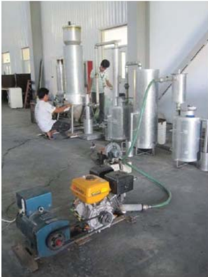
The 3-kWe Plant
