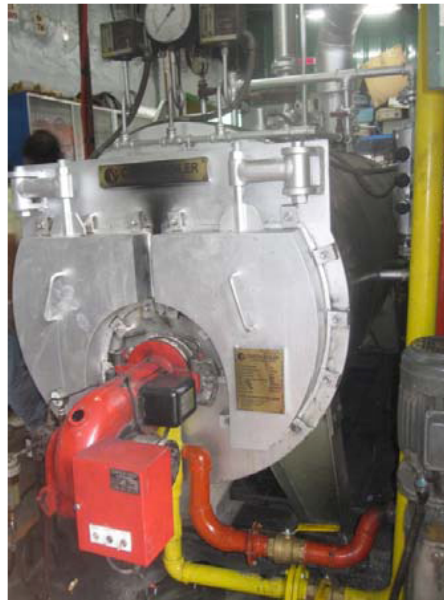
The 35-BHP Steam Boiler
