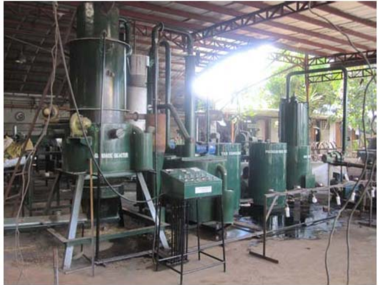
The 20-kWe Plant
