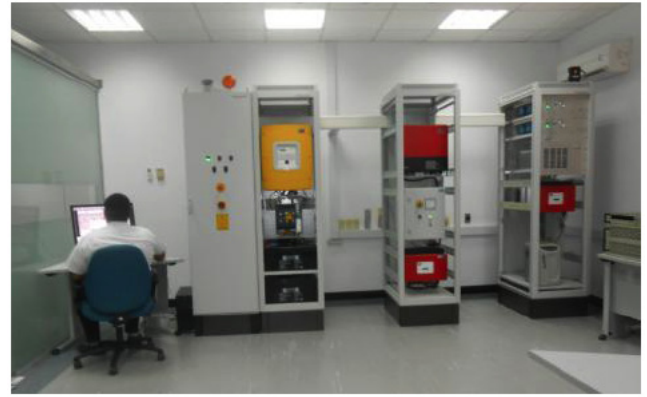
Figure 14: Center for Renewable Energy Installed at Colleges and Institutes sector of Royal Commission at Yanbu, KSA.
